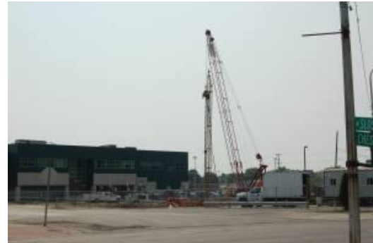
Construction of New Milk Processing Facility General Mills, Yoplait Plant Reed City, Michigan
